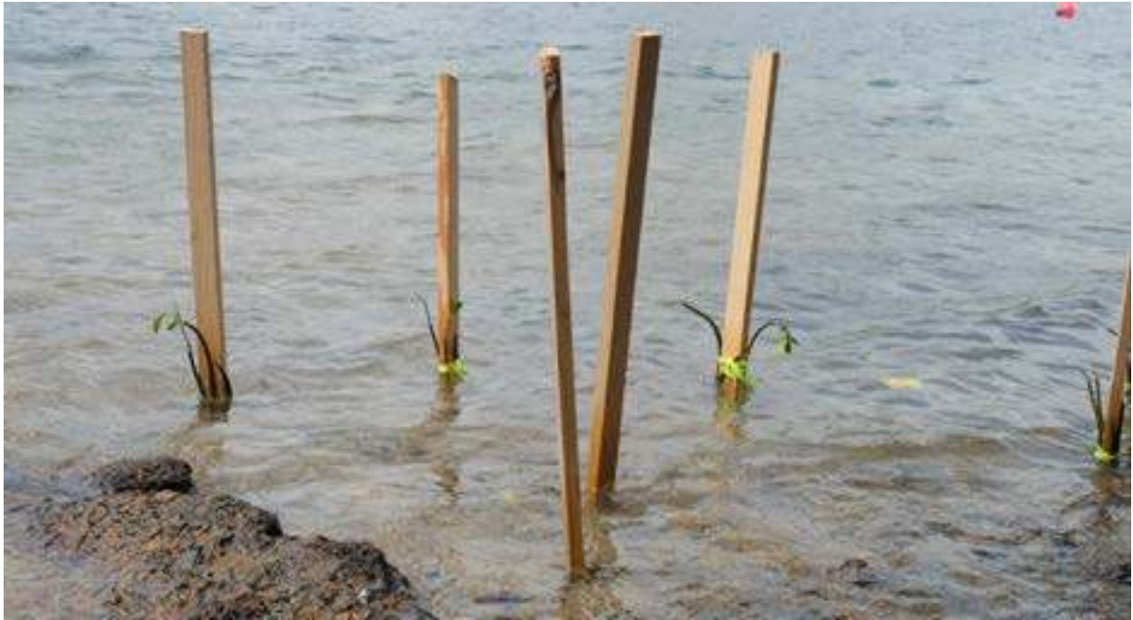
Figure 68. Planting of Ryzophora mangle propagules following Bauzá technique to anchor areas of propagules and facilitate planting establishment. (Photos courtesy of L. Medina)
