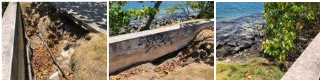
Figure 44. Eroded points along the boardwalk's retaining wall both inland and in water's edge. (Photos courtesy M. Rodríguez)
