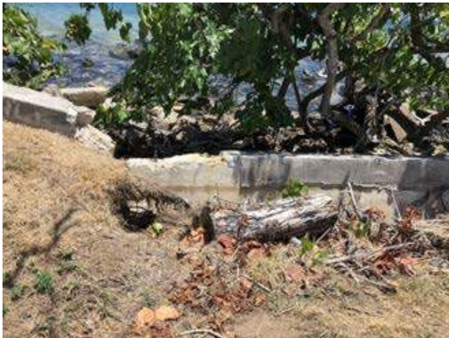
Figure 6. Eroded embankment area and partial retaining wall collapse. (Courtesy of M. Rodríguez)
